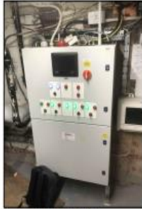
BMS CONTROL PANEL
